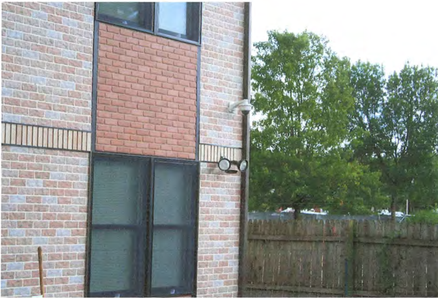
Directional lighting to provide illumination for the exterior parking area at night.
